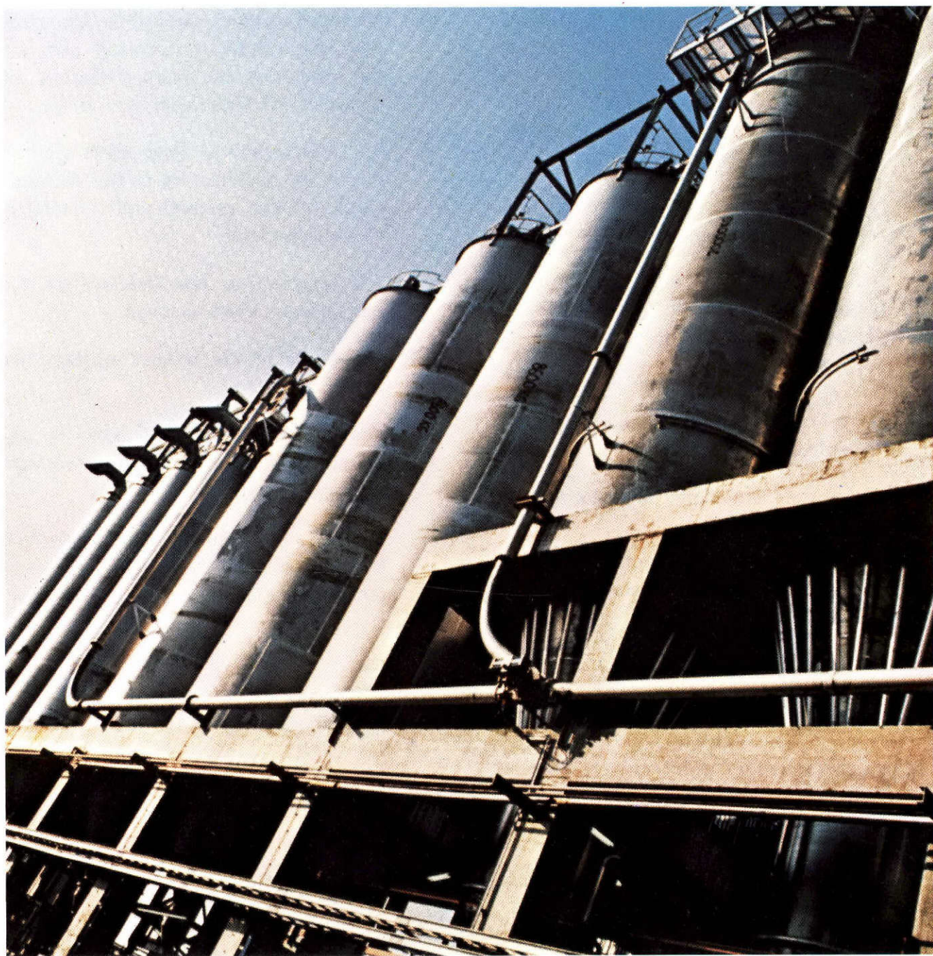
Silos for Low-Density Polyethylene Project
