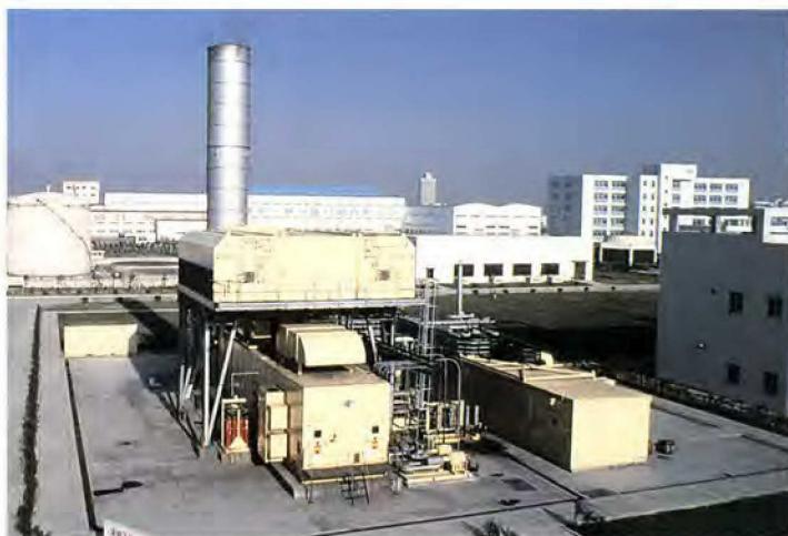
Wuxi Huada Gas Turbine Electric Power Company is providing electricity to commercial users in Wuxi City, Jiangsu Province, China.
