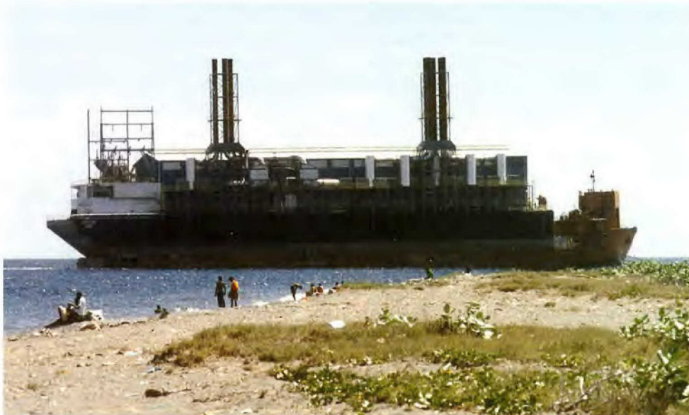
MIGA issued new coverage to this barge-mounted diesel power plant at Old Harbour, Jamaica.
