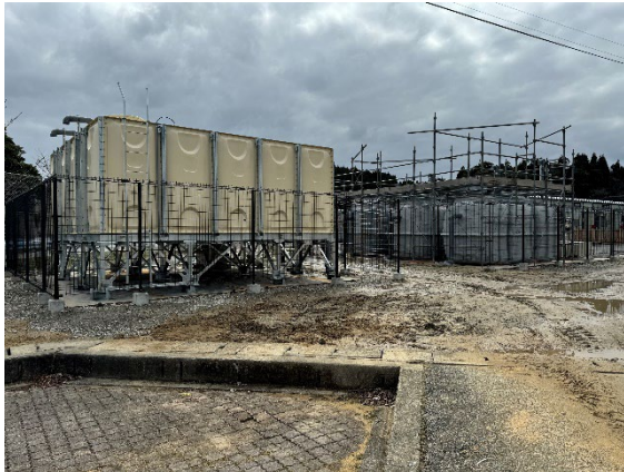
Water tank/septic tank
