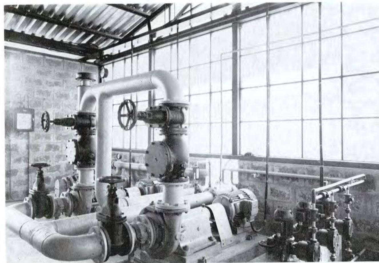
Boké Water Pumping Station.
