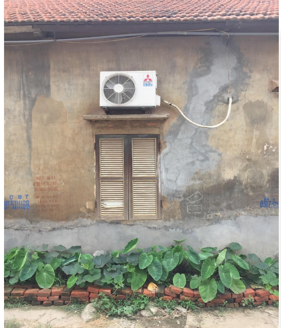
Residential AC unit in Vinh Phuc
