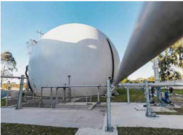
Photo: Biogas storage from anaerobic domestic sewage treatment at Atuba Sul WWTP, Curitiba, Brazil. Clean energy from methane and biomass (dried sludge and wood chips) is used to generate heat for a full scale sustainable thermal drying and combustion sewage sludge system (Credit: Sanepar).
