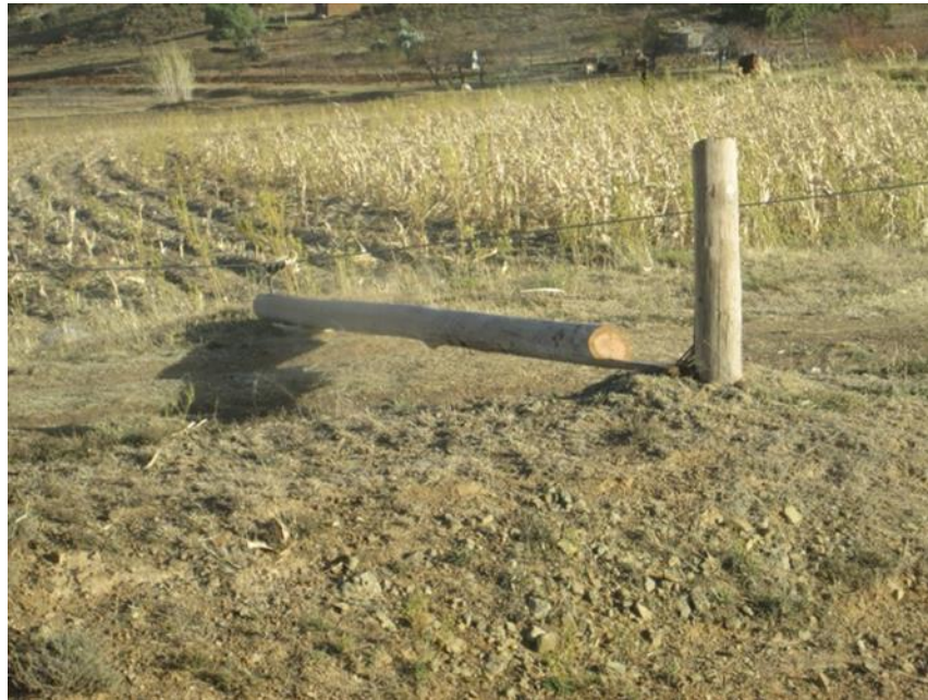
Figure 23: ETL pole on route to Mohale’s Hoek which was cut down by thieves or vandals
