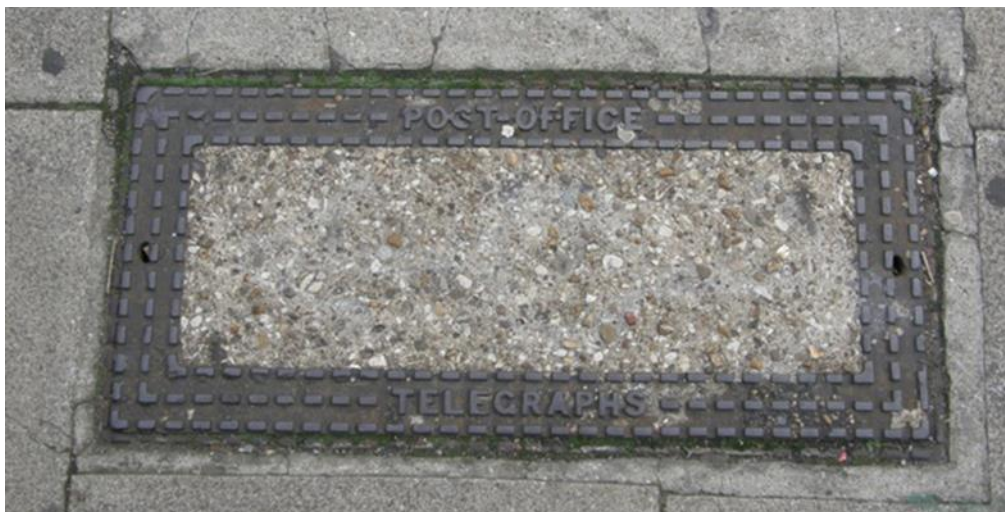
Figure 6: Access cover for buried telegraph cable in the United Kingdom
