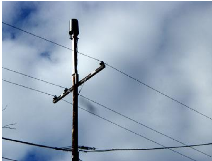
Figure 14: AT&T distributed antenna system installed atop electricity distribution pole in California
