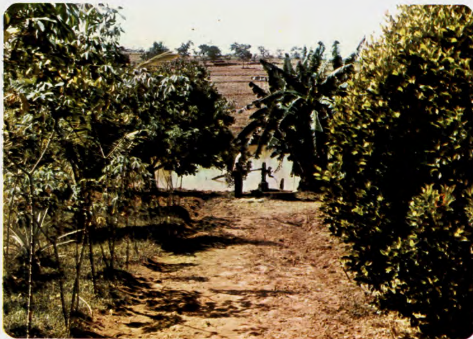
SHALLOW WELL PUMP INSTALLED NEAR EARTH DAM
