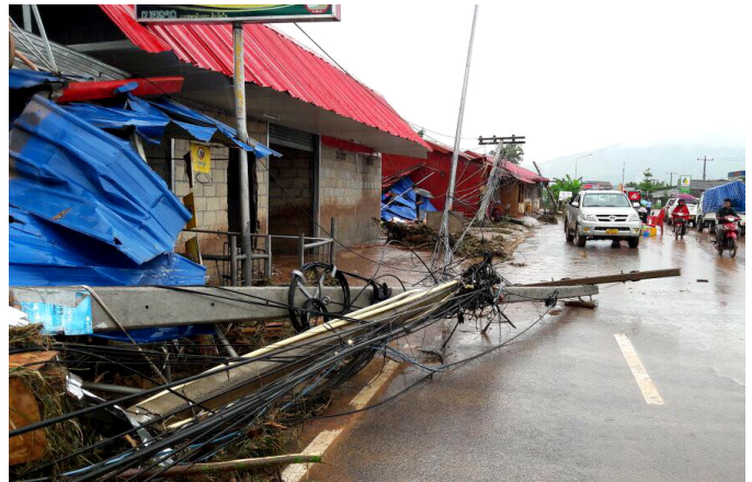
A powerline lies in the street following 2017 floods in Oudomxay, Lao PDR (Photo source: World Bank)
