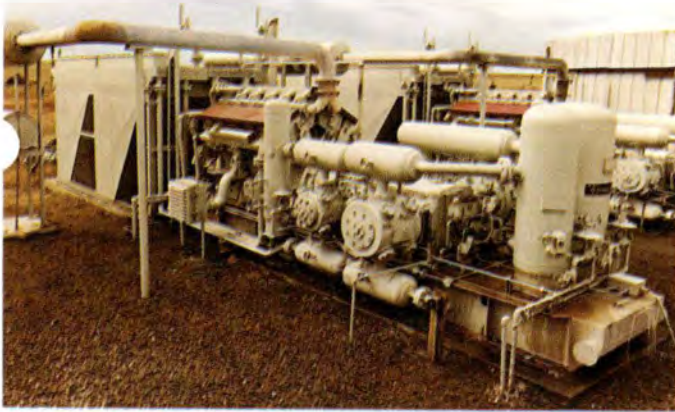
CASING HEAD GAS compressor station in western Oklahoma is on stream twenty-four hours a day unattended. Uses two five-inch (12.70 cm) stroke, four-throw, three-stage compressors operating from 20 psig (1.41 Kg/cm 2 ) to 900 psig (63.28 Kg/cm 2 ).
