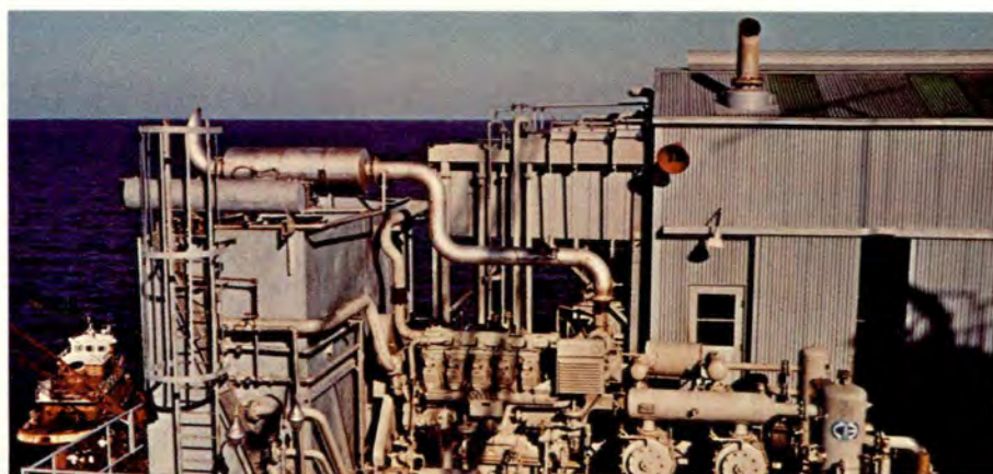
FLARE GAS operation on this platform one hundred miles (160.93 KM) off the Louisiana coast uses a six-inch stroke (15.24 cm), four-throw, three-stage "FE" compressor at 1200 psig (84.37 Kg/cm 2 ) discharge. The unit is rated at 1100 HP.
