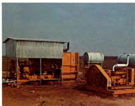
SALES GAS installation in Texas uses a five-inch (12.70 cm) stroke, two-throw "FE" compressor operating in conjunction with an eleven-inch (27.94 cm) stroke Chicago Pneumatic T-type compressor.
