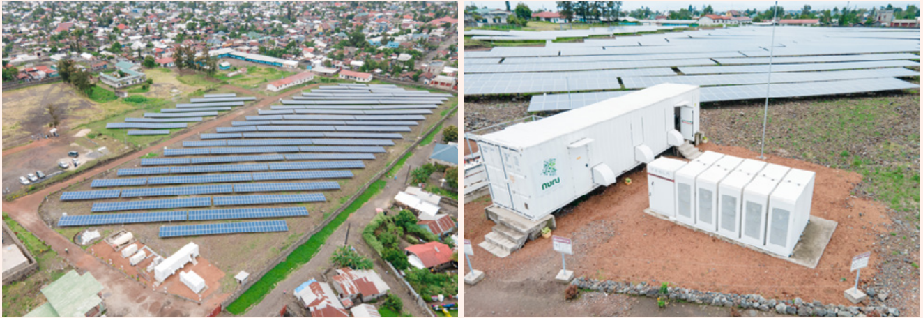
Photo 5.1. Nuru site. Located in the neighborhood of Ndosho in Goma, DRC. The site is equipped with more than 3,700 solar pannels and has an installed capacity of 1.3 megawatt
