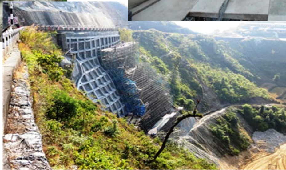
Slope Protection Works at Sindhuli Road, National Road No.6 Nepal in 2014 through a Japanese Grant (JICA)
